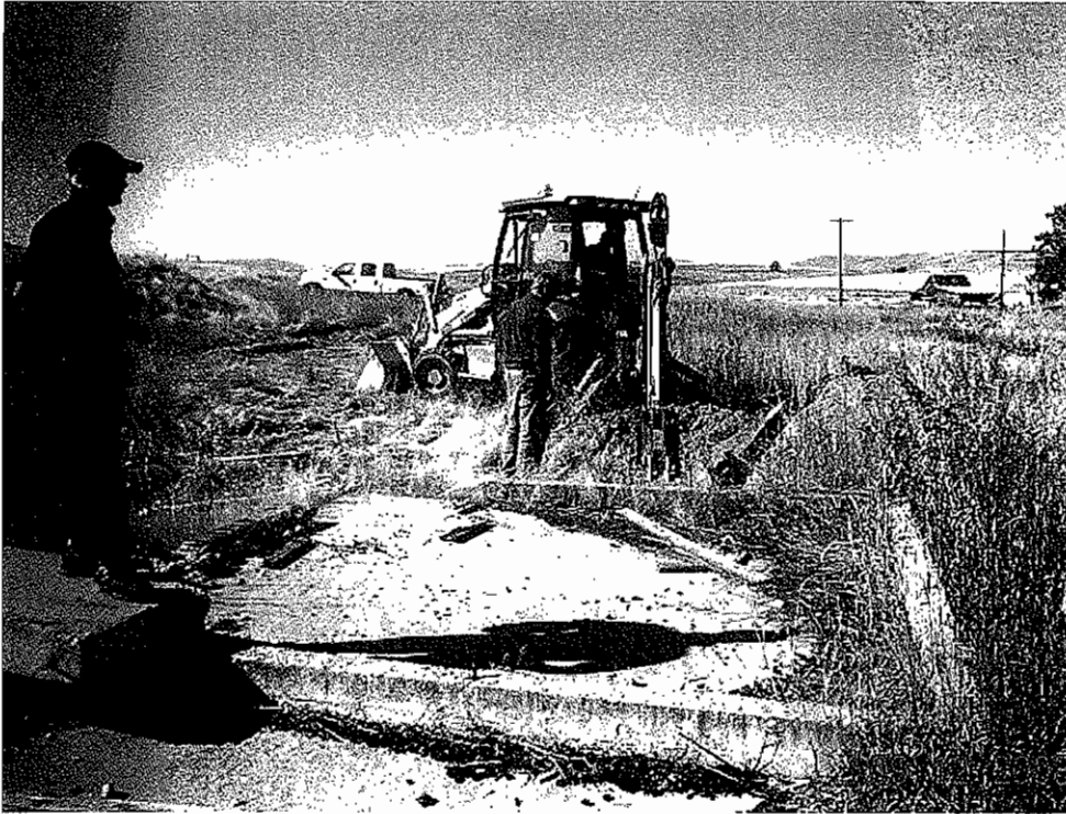
Cement pad near test pit No. 8, west of main site, looking south
